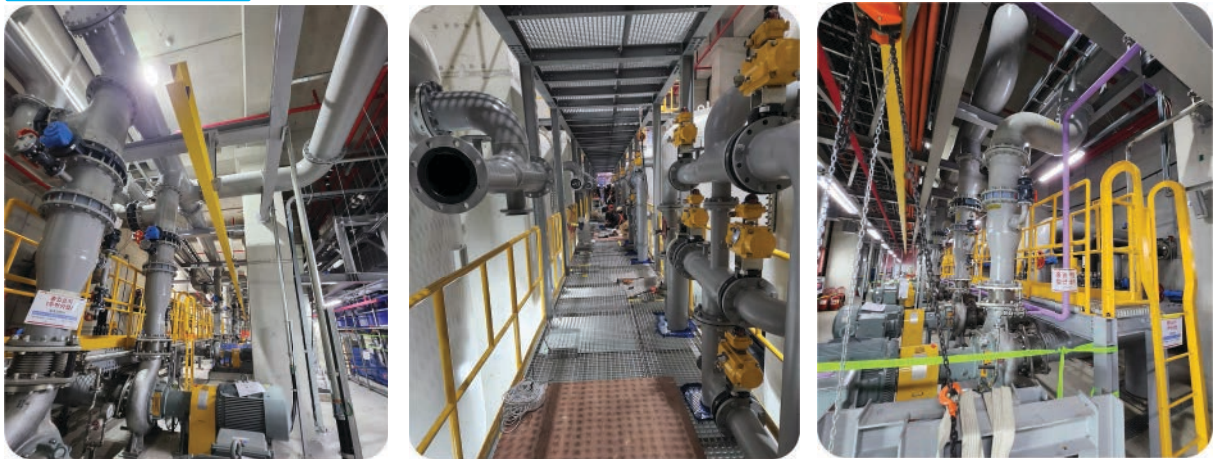
▶ Water treatment equipment piping (Factory)
