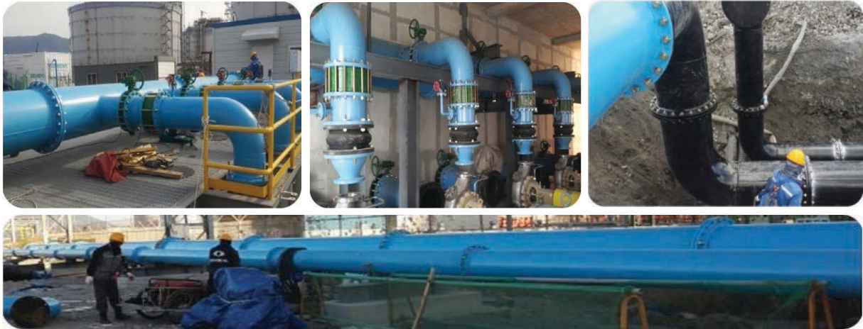
▶ Seawater desalination facility piping and LNG terminal piping
