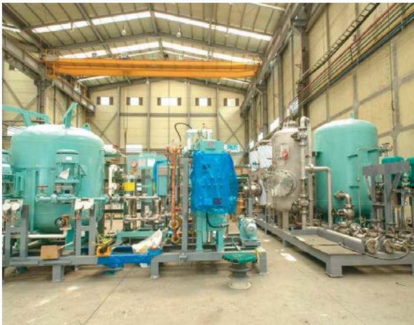
Fresh Water Supply Plant
