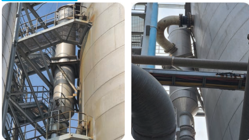
▶ Methane gas storage
