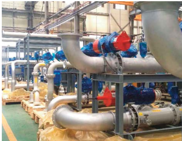
Front Pipe Skid
